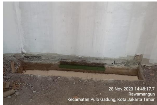
Gambar 4. Void area Ruang Panel Proyek UNJ
