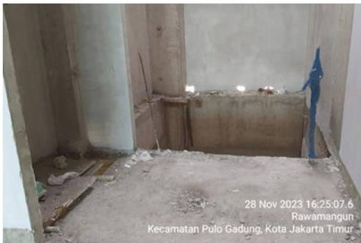
Gambar 3. Void area Lift Service Lantai 3 Proyek UNJ
